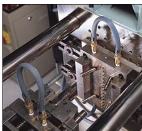
▲ For coolant piping for molds
