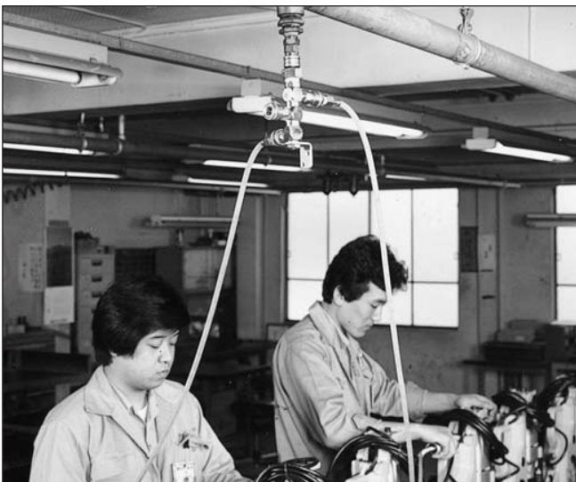
▲ Air pipe branching
